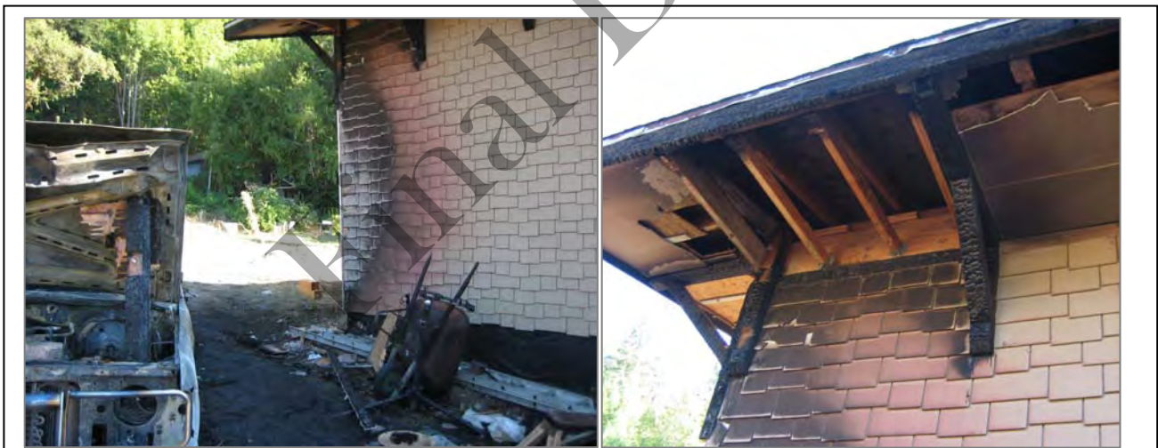
Photo 4-1: The photos above show damage that took place to a rural West County home when the vehicle on the far left ignited (cause undetermined). Highly aware of the wildfire risk in their area, the homeowners had recently replaced wooden siding with fiber-cement shingles, and enclosed the soffit with fiber cement sheathing. They also have well-maintained defensible space. The fire burned for at least one-half hour before firefighters were notified and arrived on the scene. Due to intense heat from the vehicle, there was some fire intrusion into the attic space which had to be repaired. However, if the residents had not taken action to replace flammable siding, it is likely that the home would have been a total loss. Likewise, their good defensible space kept the fire from spreading into the surrounding wildland.
