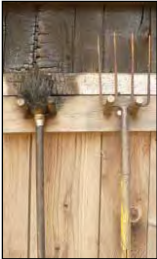
Though it charred the siding, luckily, the broom didn't fully ignite this building.
