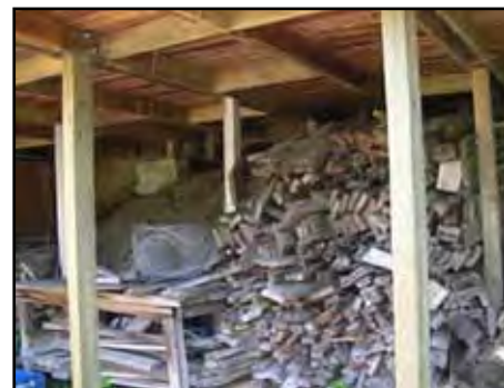
If items stored under the deck can ignite from embers, deck and structure will follow along. Don't store combustibles under decks!
